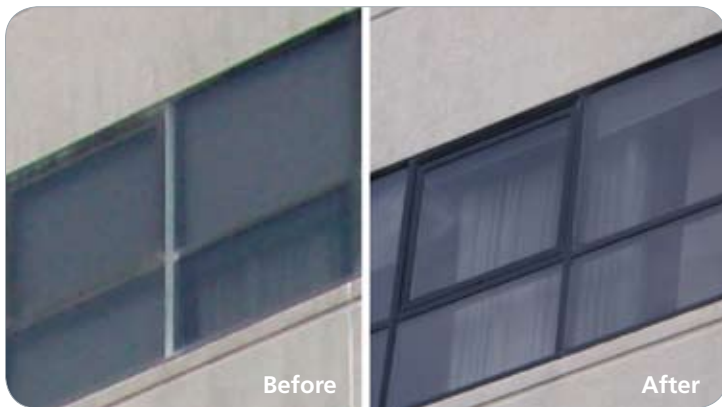
Valcourt recently completed mullion cleaning and coating for the Sheraton Eatontown Hotel in New Jersey, which returned luster and color to its mullions.
